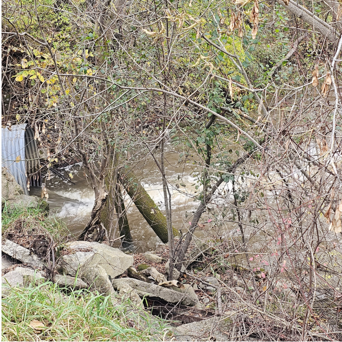
Photo 3: Undersized culvert on Angier Hill Rd.
