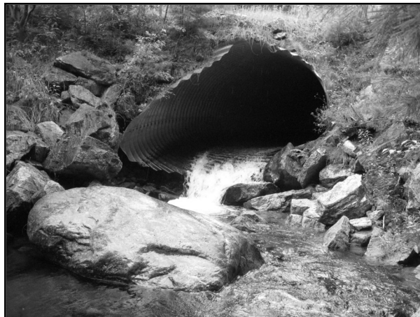
This culvert, on Spruce Mill Brook in Lewis, would open up approx. 9 miles of streams if retrofitted.
