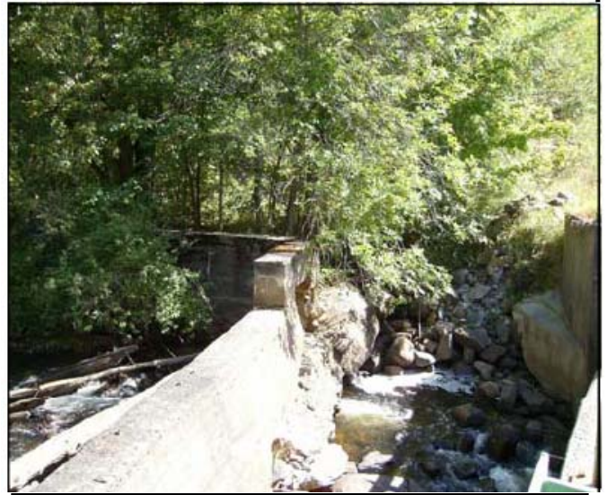
The Crowningshield Dam prior to being removed. Picture courtesy of Essex County SWCD
