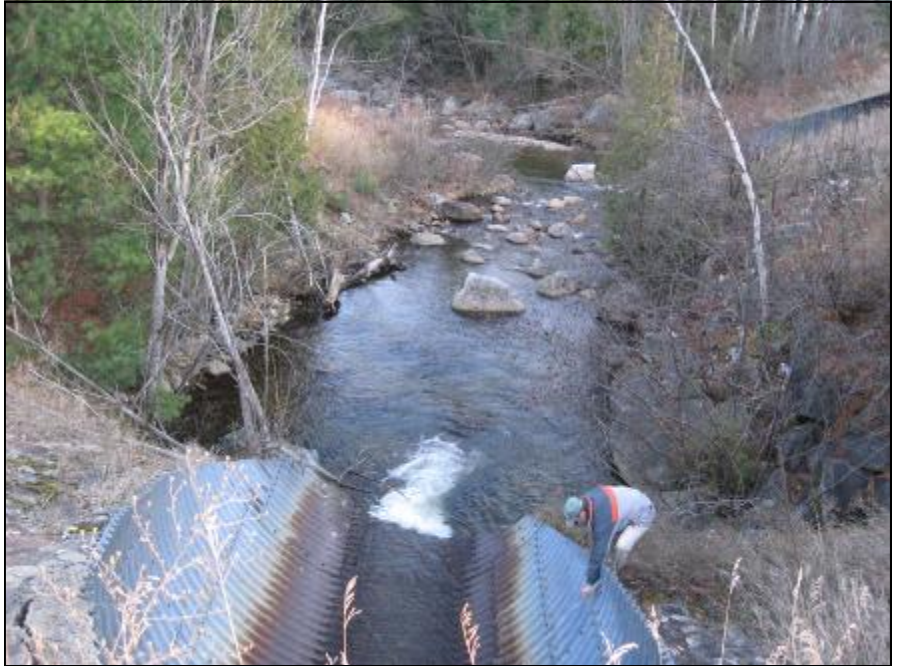
This culvert, where Slide Br. joins The Branch in Elizabethtown, has an 8+-inch vertical drop.
